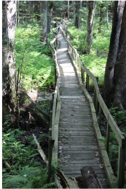
The previous Hi-Lo Bridge In Poor Condition Prior to Removal
