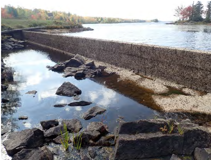
Picture 2.0 – Deerock Spillway. Showing exposed rebar, cracking and worn concrete.
